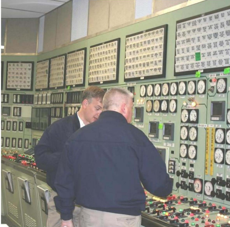
Operators review procedures in the control room while putting St. Lucie Unit 2 online following a refueling outage.
